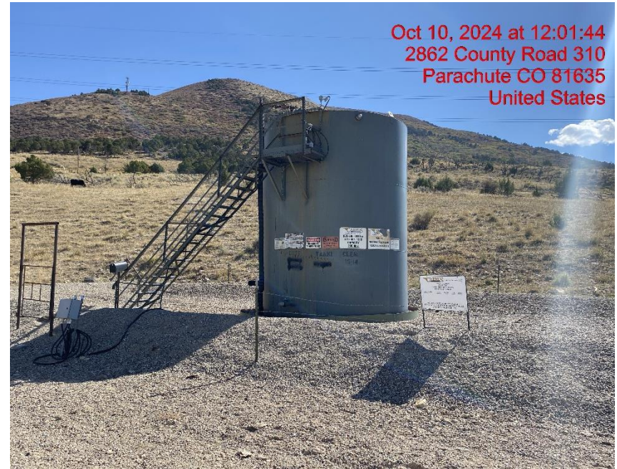
Tank Battery – Photo #04147
