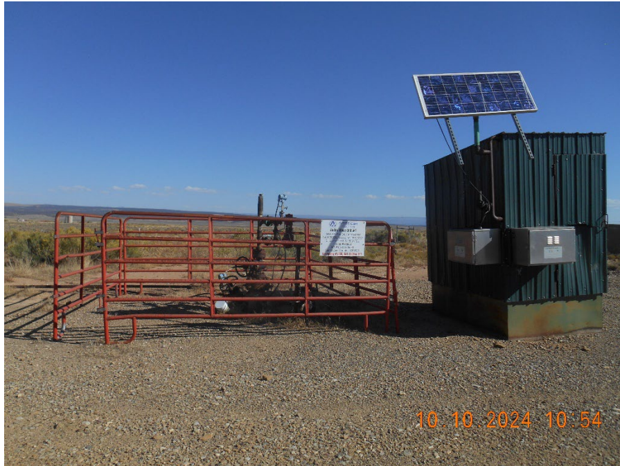
Wellhead with fence and sign
