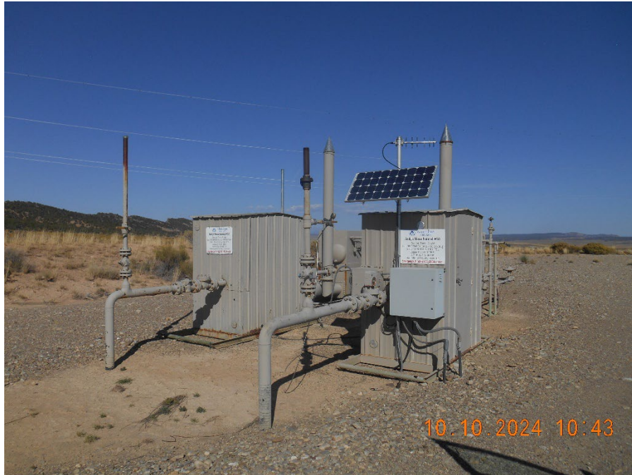
Separators and Meter housings
