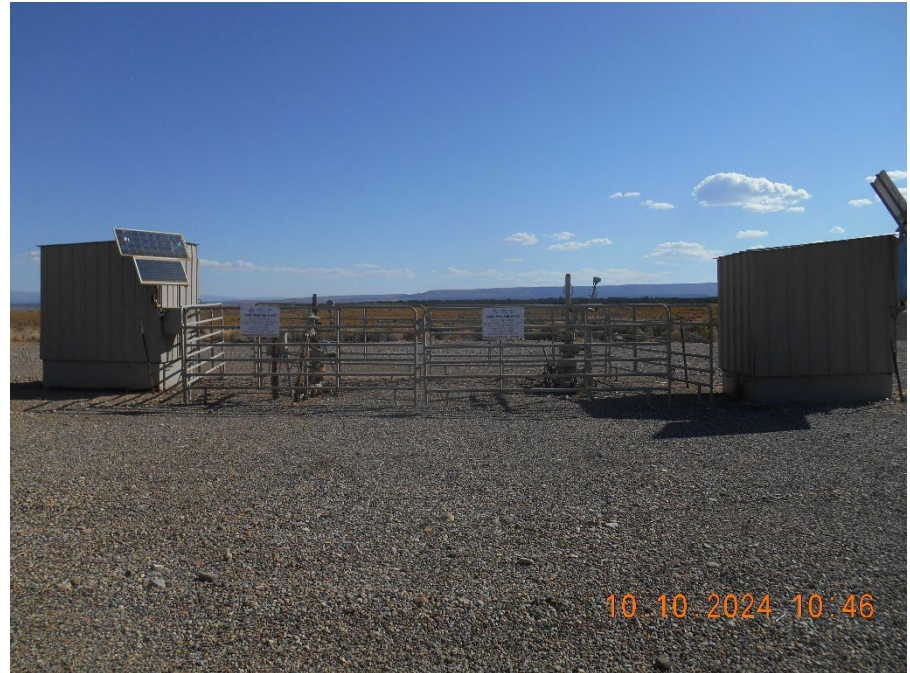
Wellheads with fence and signs
