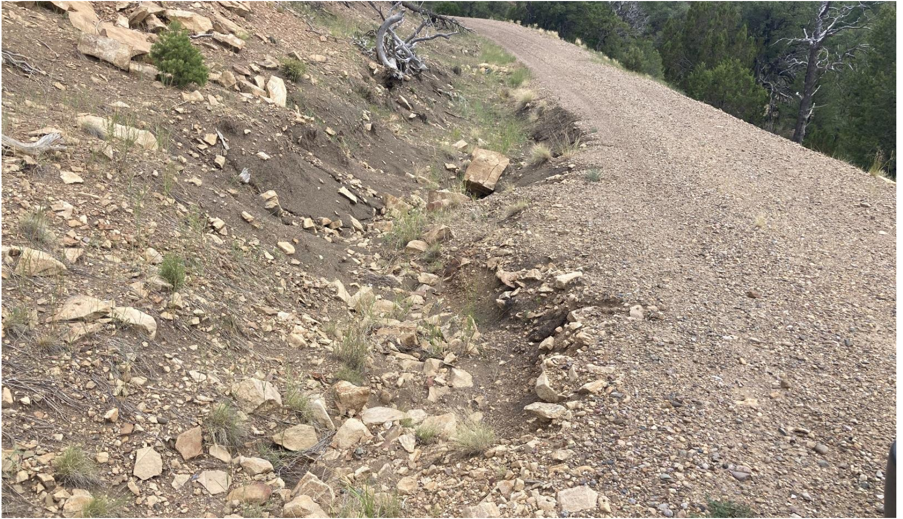
PHOTO 6: PHOTO FROM PREVIOUS INSPECTION TAKEN ON 8-3-2023.
