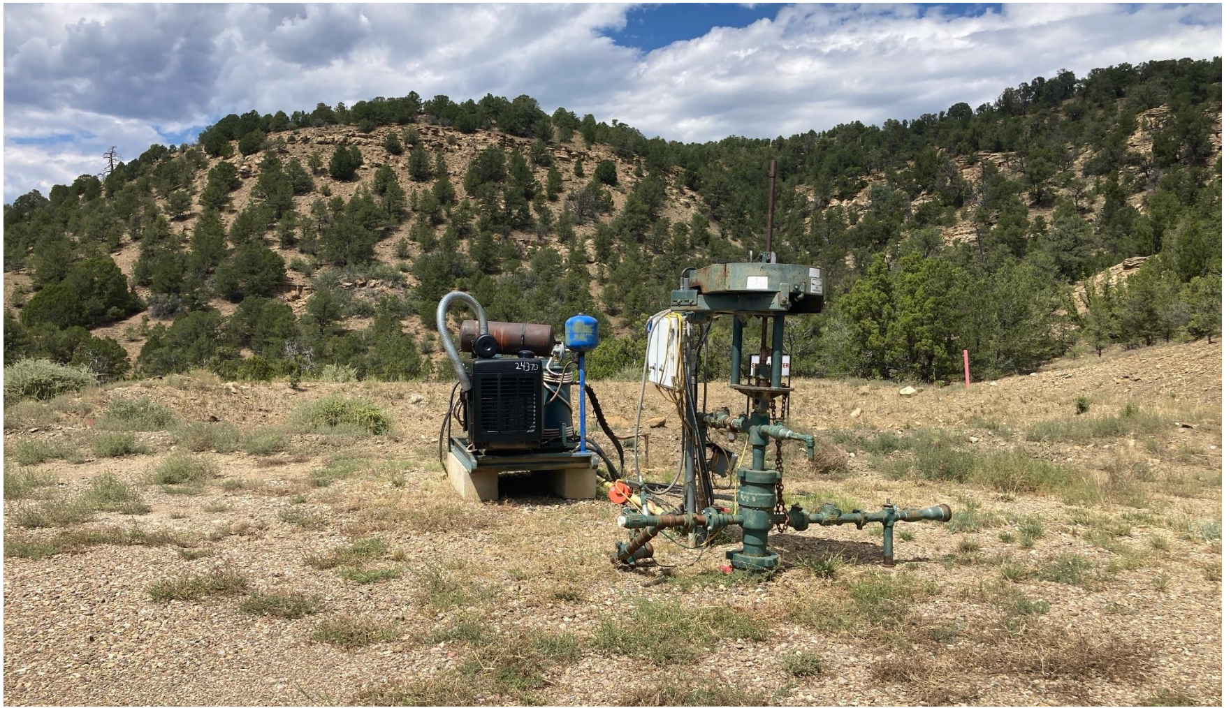
PHOTO 3: WELLHEAD AND EQUIPMENT
