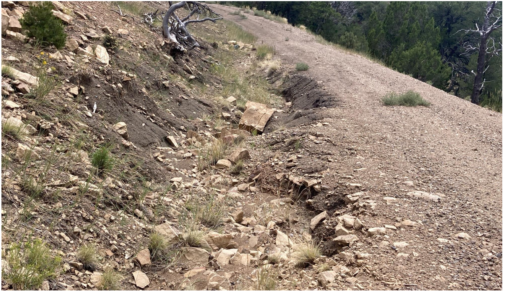
PHOTO 5: STORMWATER IS WASHING OUT DITCH AND ERODING INTO THE ROW EAST OF LOCATION. INSTALL STORMWATER PREVENTION AND MAINTAIN ACCORDING TO RULE 1002. THIS IS THE SECOND NOTICE FOR THIS CORRECTIVE ACTION, IMMEDIATE ACTION IS REQUIRED.
