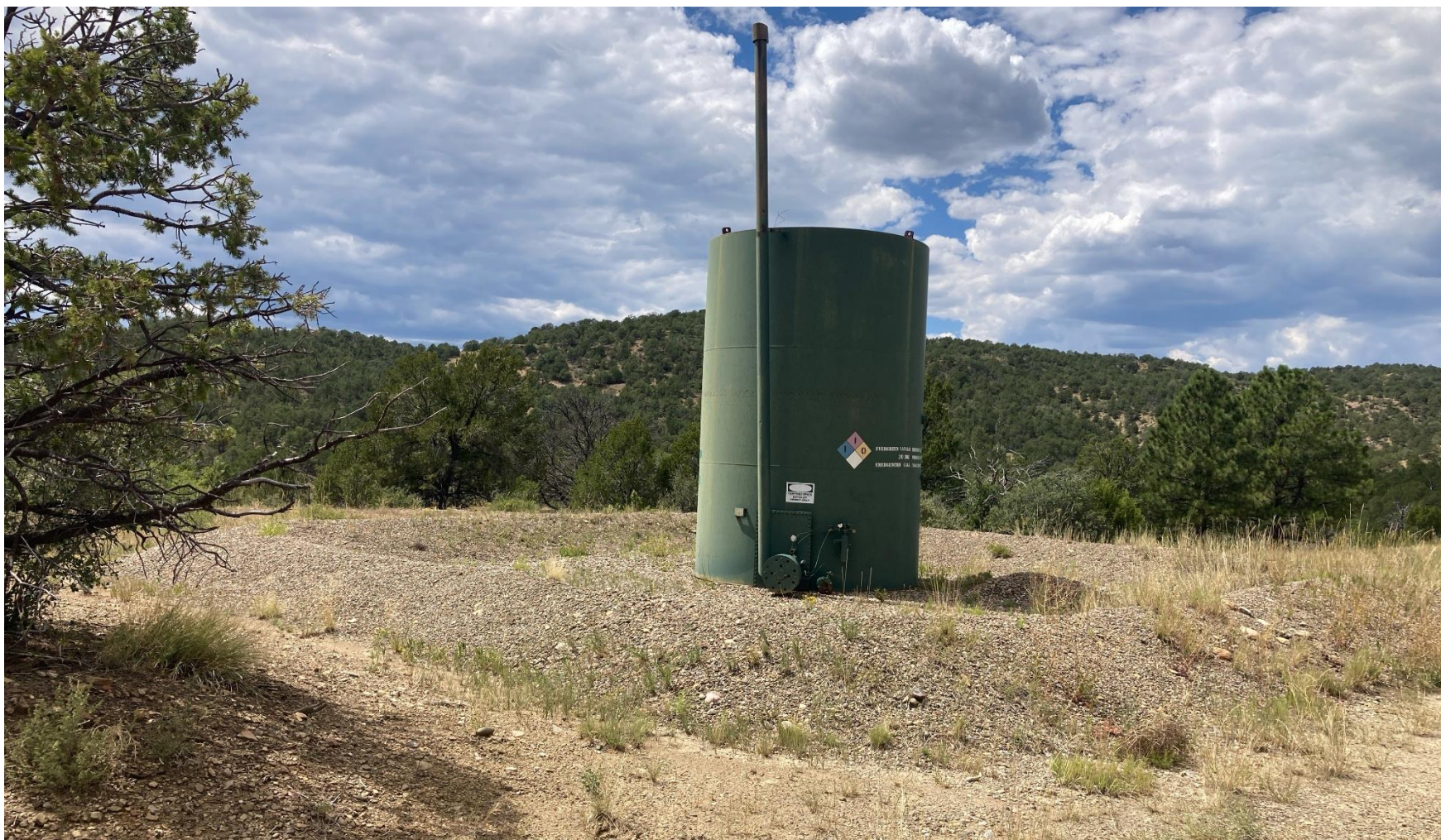
PHOTO 4: PRODUCED WATER TANK BATTERY.
