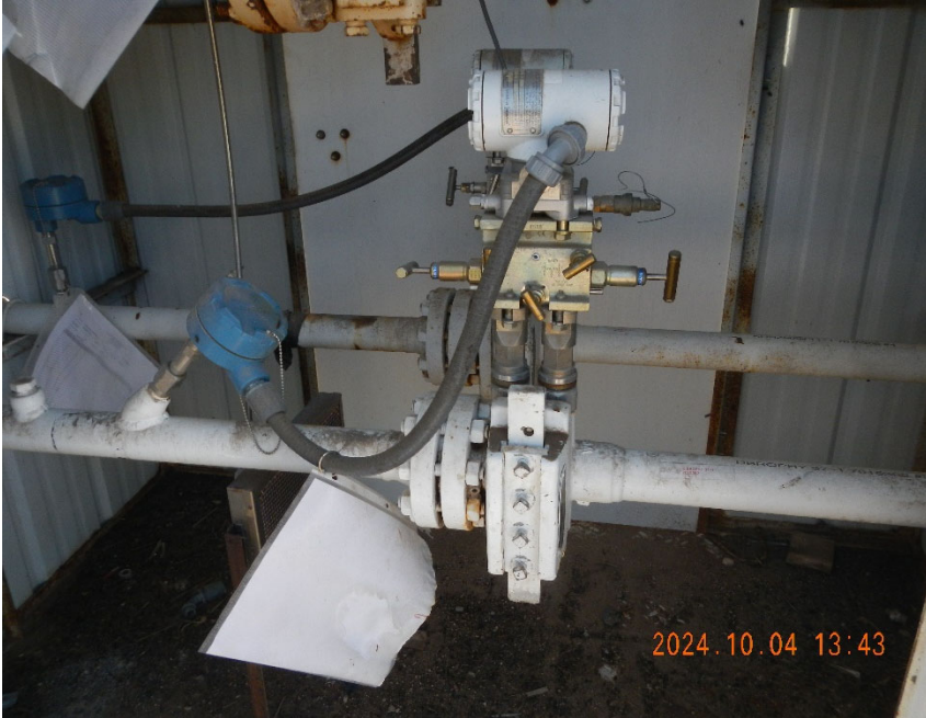
5. Gas meter inside shared meter shed.
