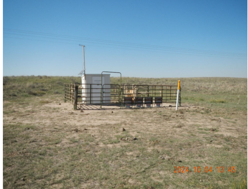
6. Remote battery location overview.
