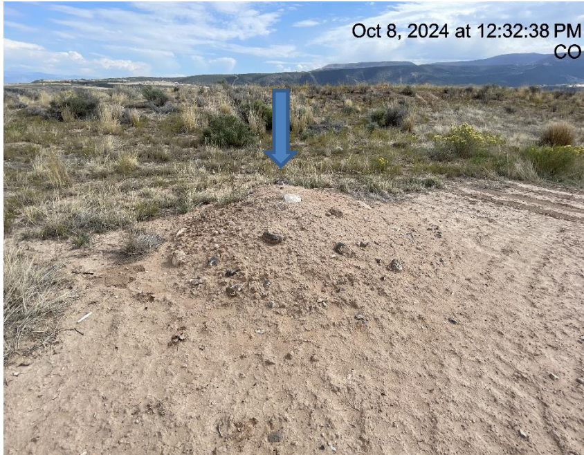
Photo # 4029 Small soil stockpile with no BMP's
