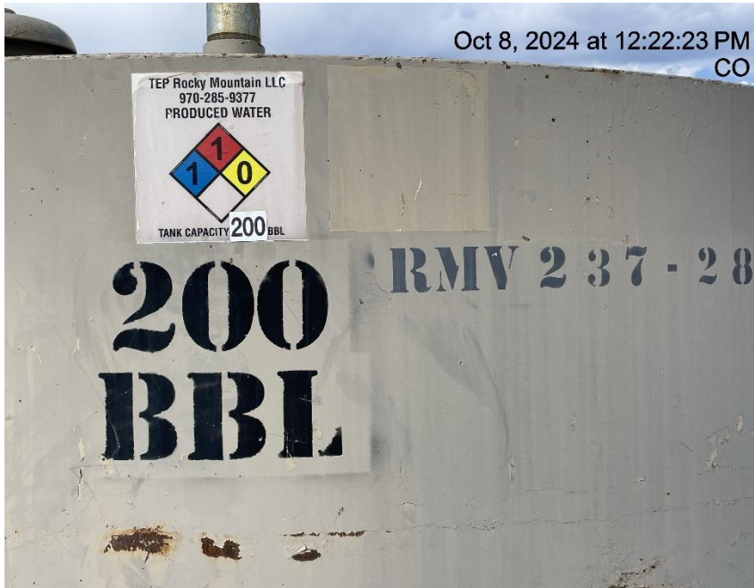
Photo # 3983 Production tank labeled inaccurately/capacity incorrect
