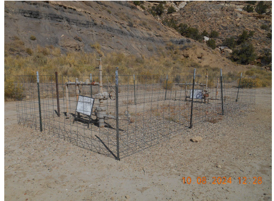
Wellheads with signs and fence
