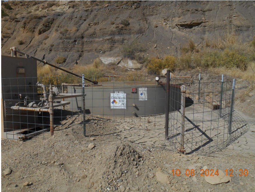
Tank battery with signs and fence
