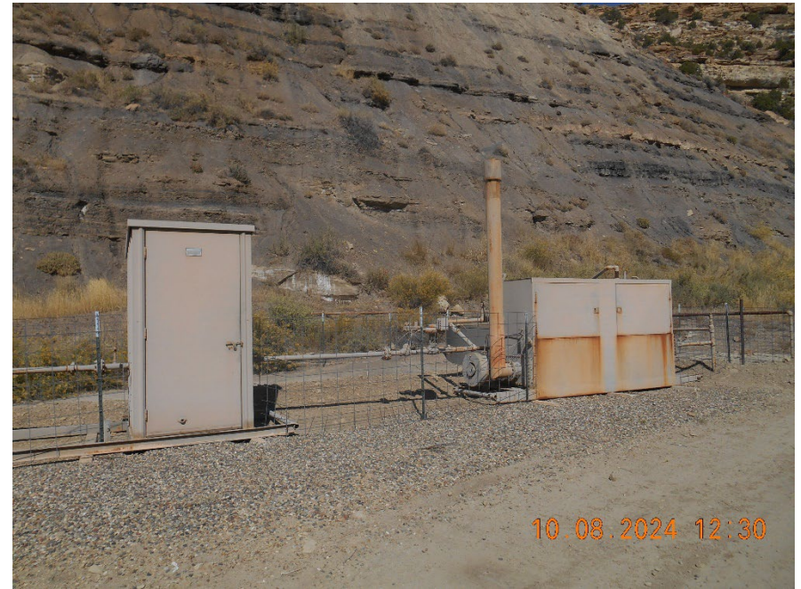
Meter housing and Separator with fence
