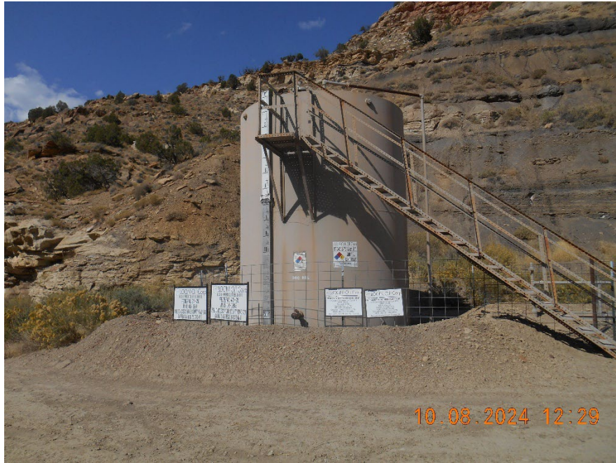
Tank battery with signs and fence
