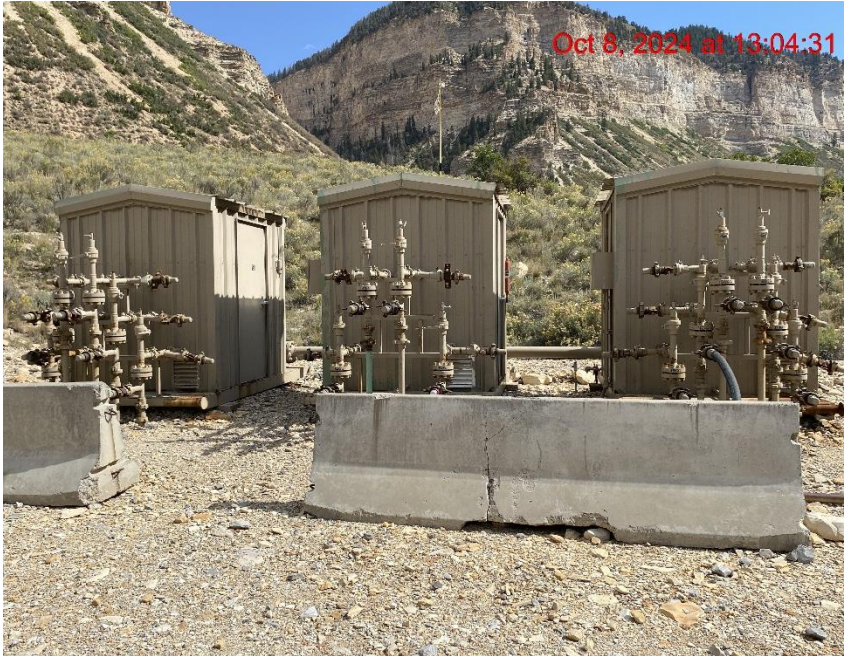
Gas Meters – Photo #04003
