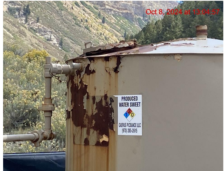
Peeling Paint/Corrosion – Photo #04005
