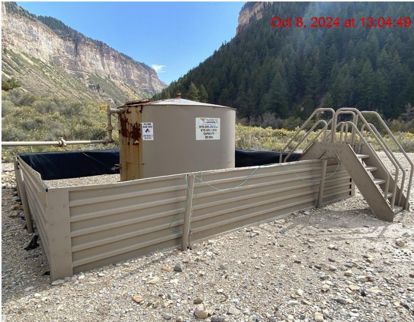
Tank Battery – Photo #04004
