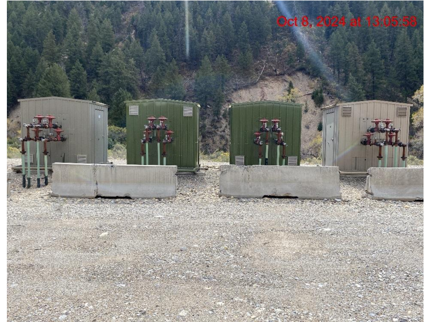
Gas Lift – Photo #04008
