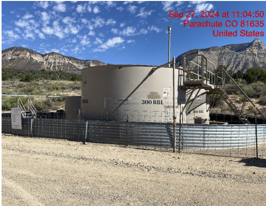
Tank Battery – Photo #03857
