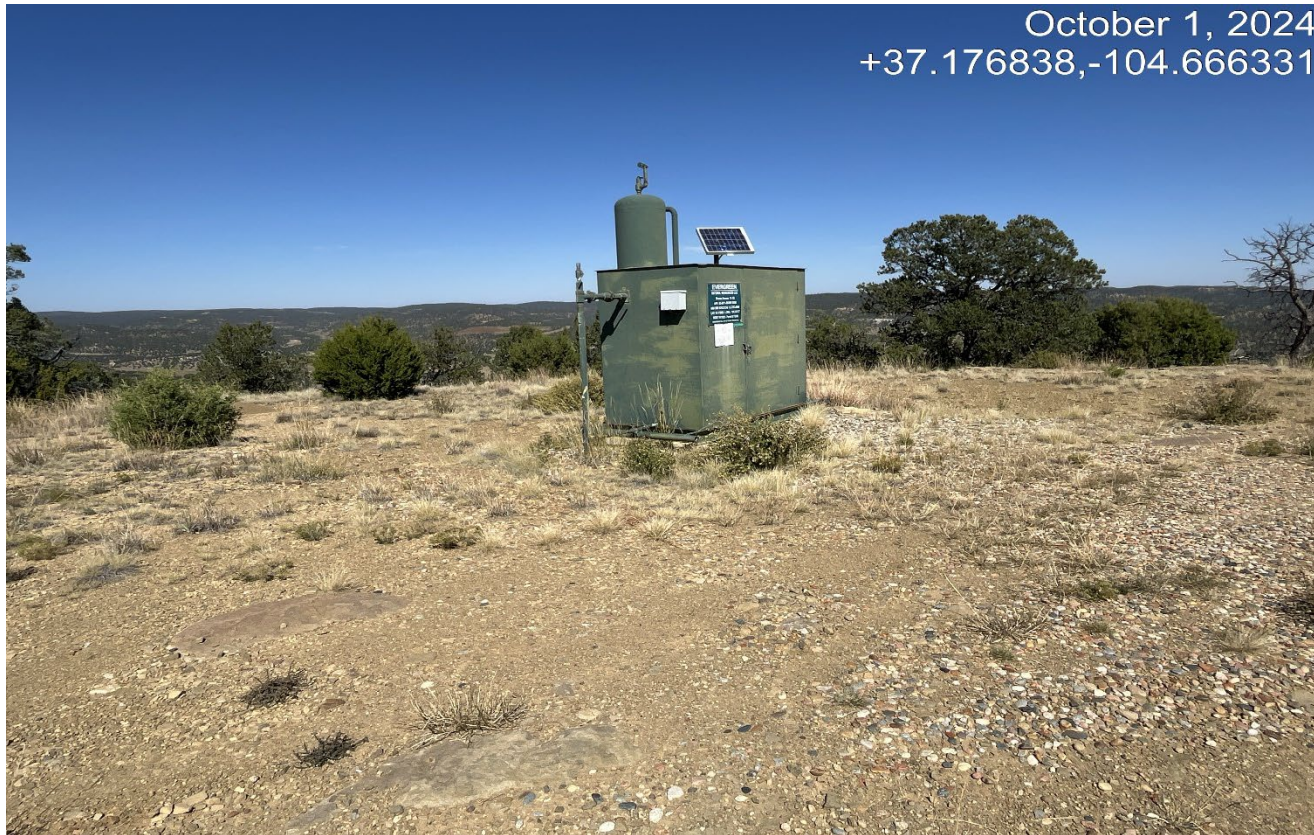
Photo 2. Well sign is posted at meter shed..
