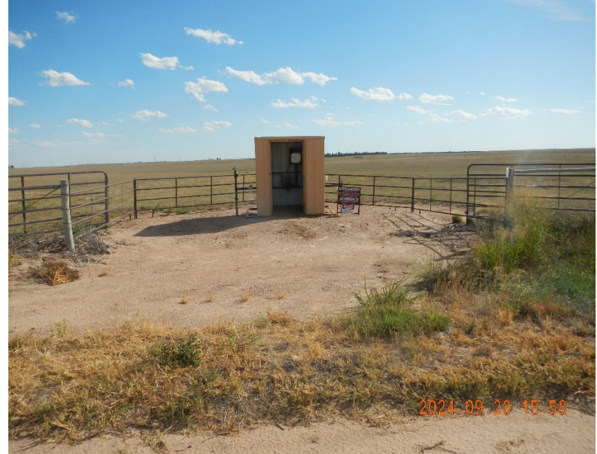
6. Remote metering location overview.
