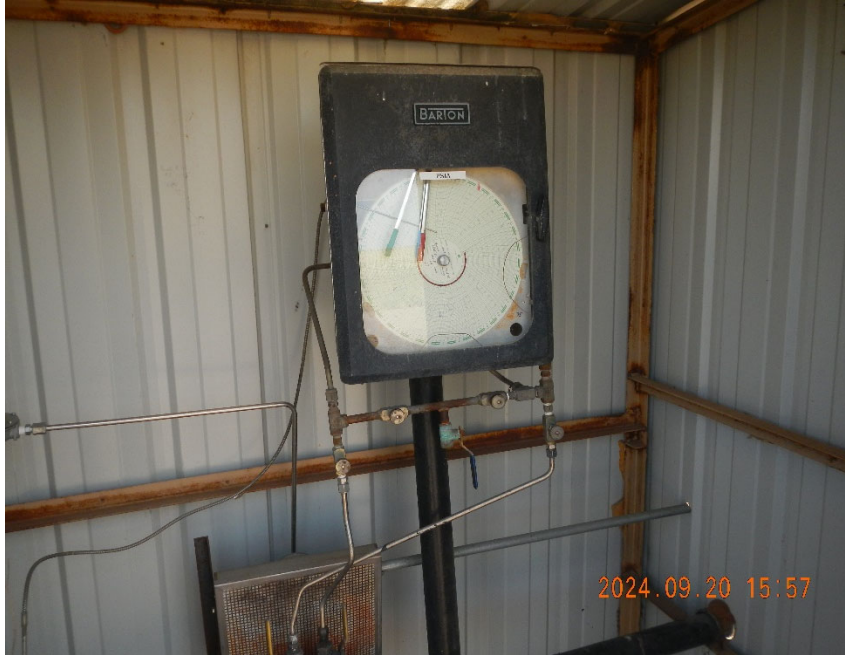
5. Gas meter inside meter shed.
