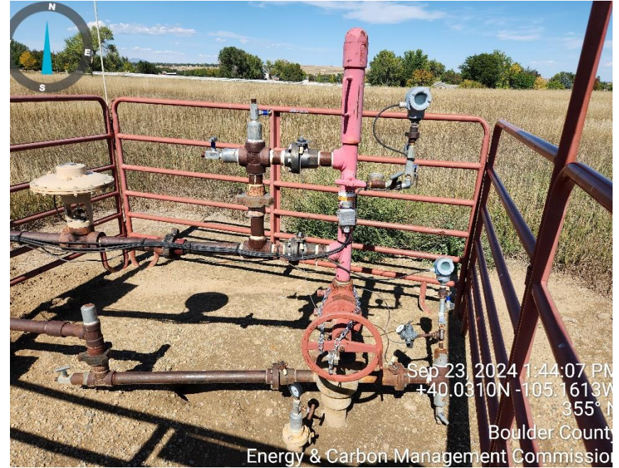
Photo 2 well head and equipment
