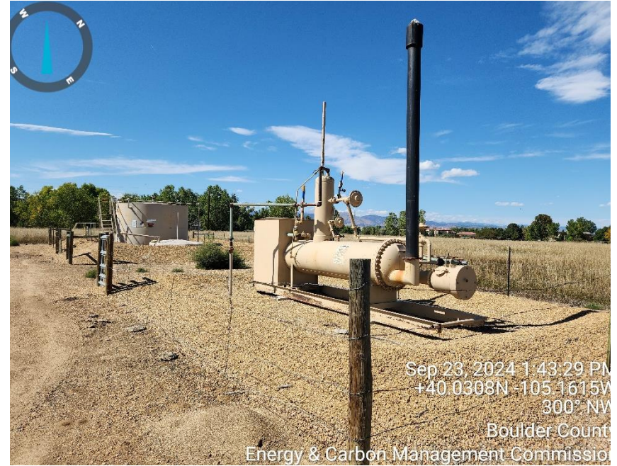
Photo 4 production equipment, tank battery
