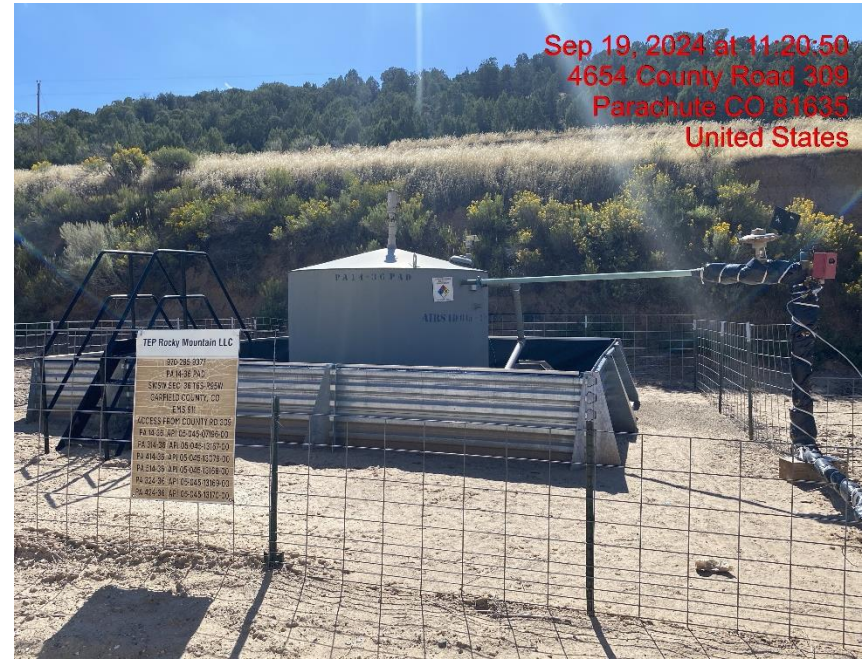
Tank Battery – Photo #03503
