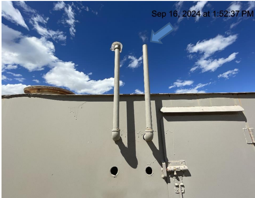
Photo # 531 PRV vent line does not comply with CECMC pressure safety device rules
