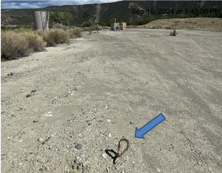
Photo # 529 Unmarked deadman
