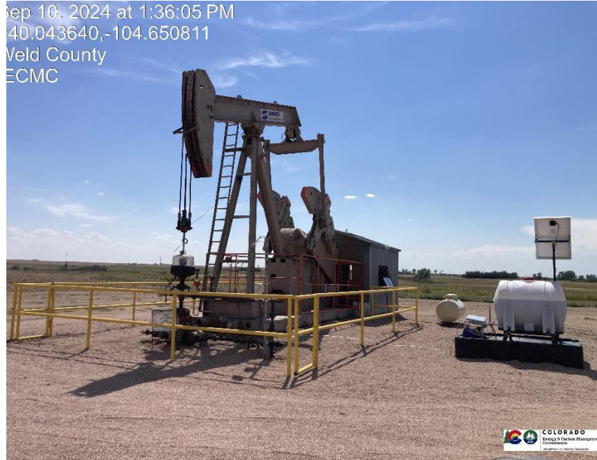
Pic 1 wellhead / pumpjack
