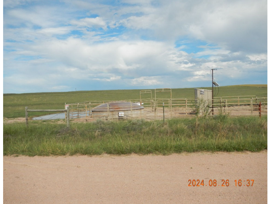
6. Remote battery location overview.
