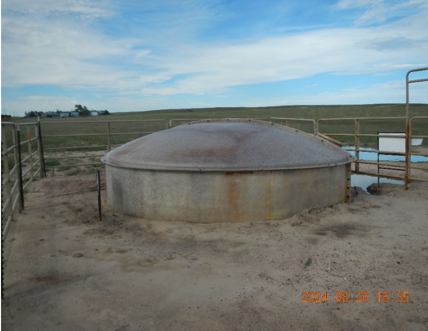
5. Produced water tank at remote battery.
