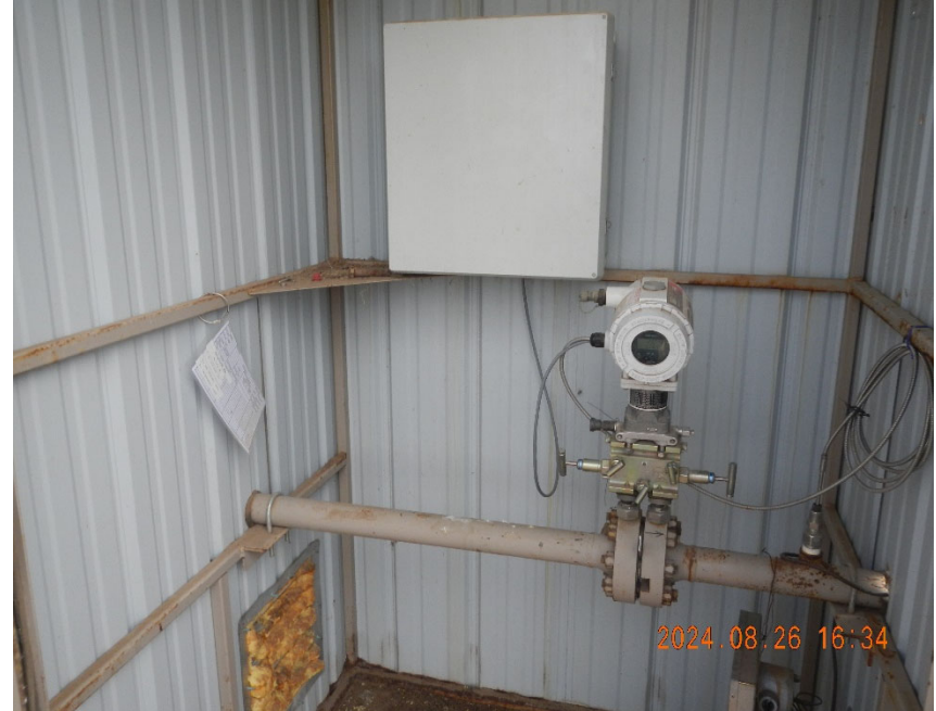
4. Gas meter inside remote meter shed.
