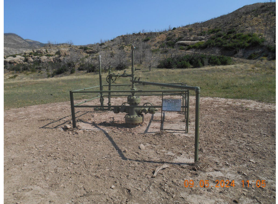
Wellhead with sign and fence
