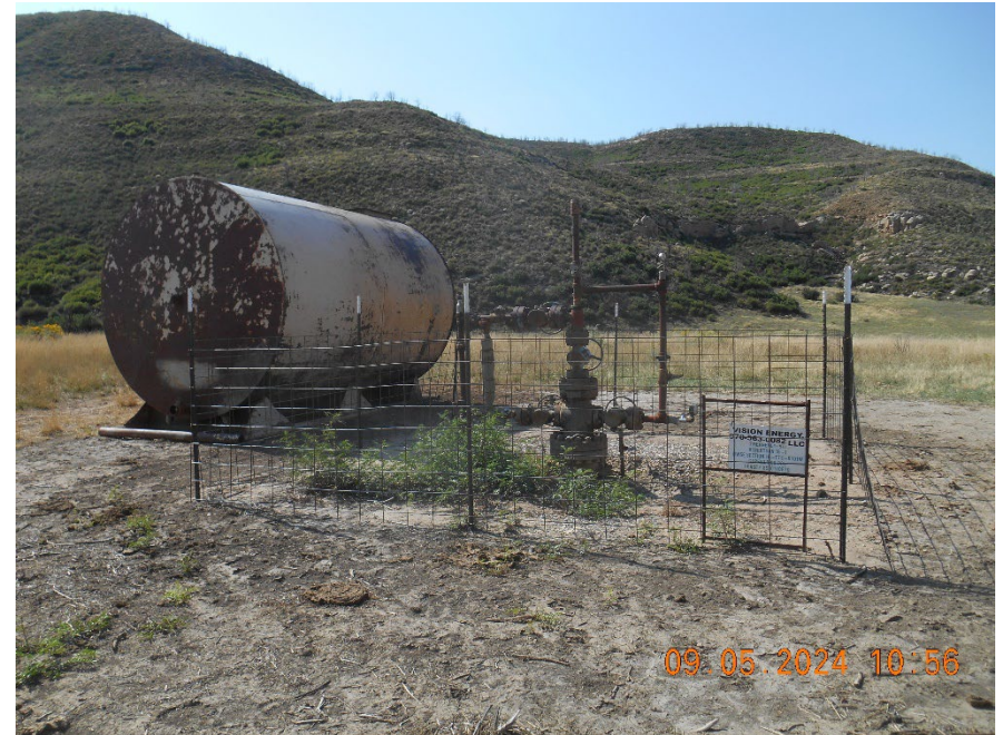
Wellhead with sign. Tank with unknown contents.
