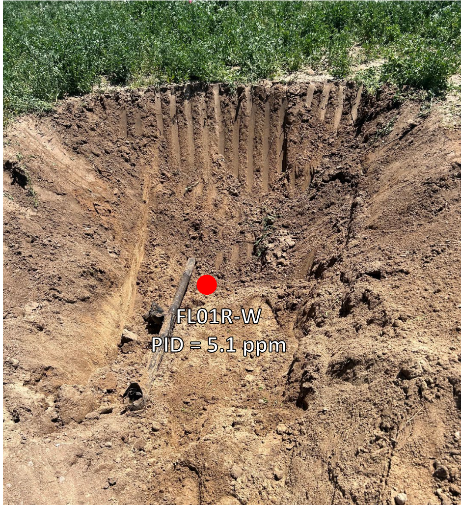
Looking north at flowline Pt A/terminus at wellhead No petroleum hydrocarbon staining or odor observed
