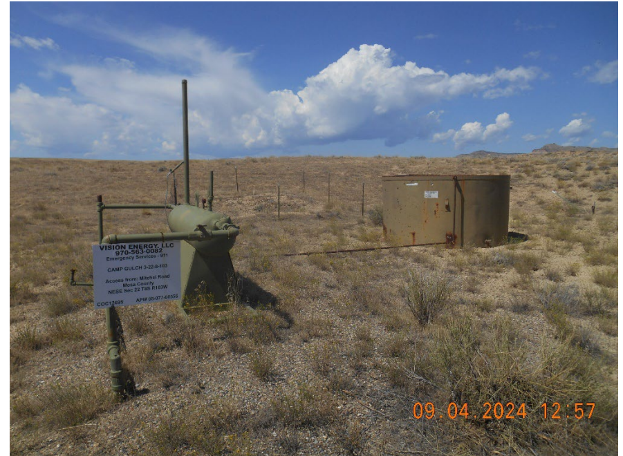
Separator with sign. Tank battery
