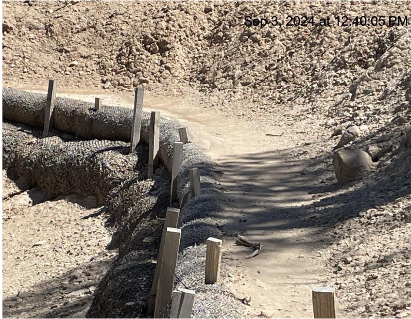
Photo # 7797 Large amount of sediment building up at waddles on slopes around tank battery/may need maintenance in near future
