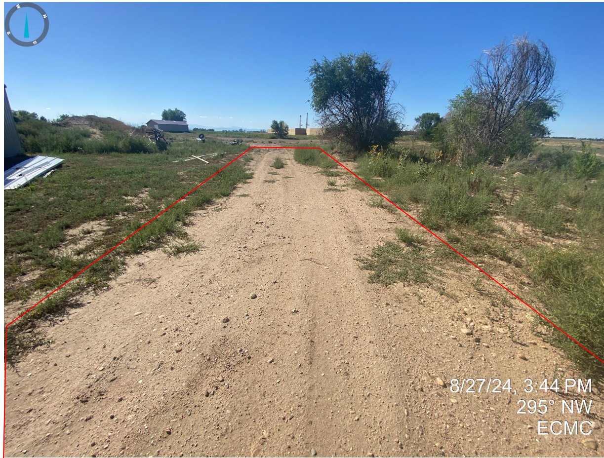
Photo 1. Facing northwest from the start of the access road. The access road does not appear to have been reclaimed with evidence of road base material observed.
