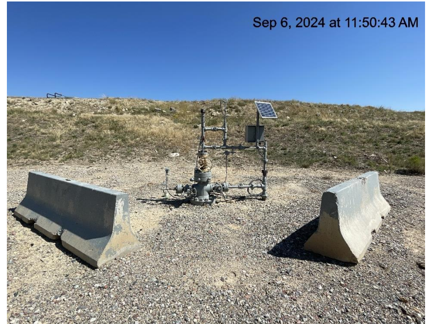
Photo # 8602 Wellhead lacks required signage/does not comply with CECMC rules
