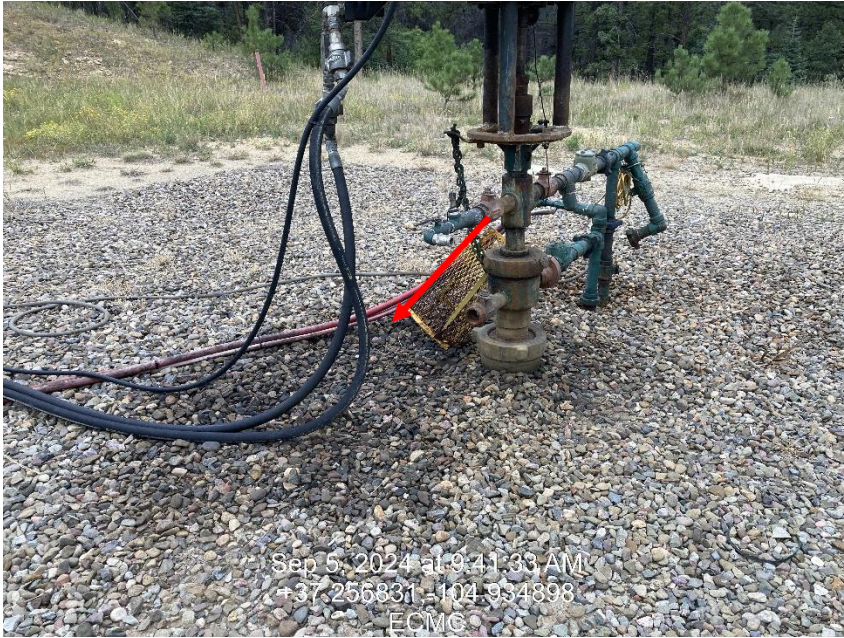
Photo 3 – Stained soils at wellhead
