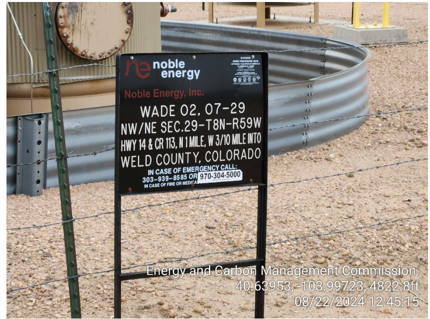
Photo 8 – Tank Battery Sign
