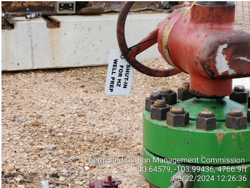
Photo 5 – Tag on Master Valve
