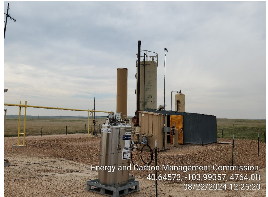
Photo 2 – Nitrogen Tank and Heater Treater
