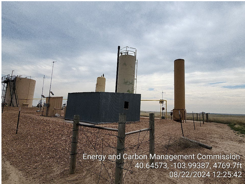
Photo 3 – Heater Treater and ECD
