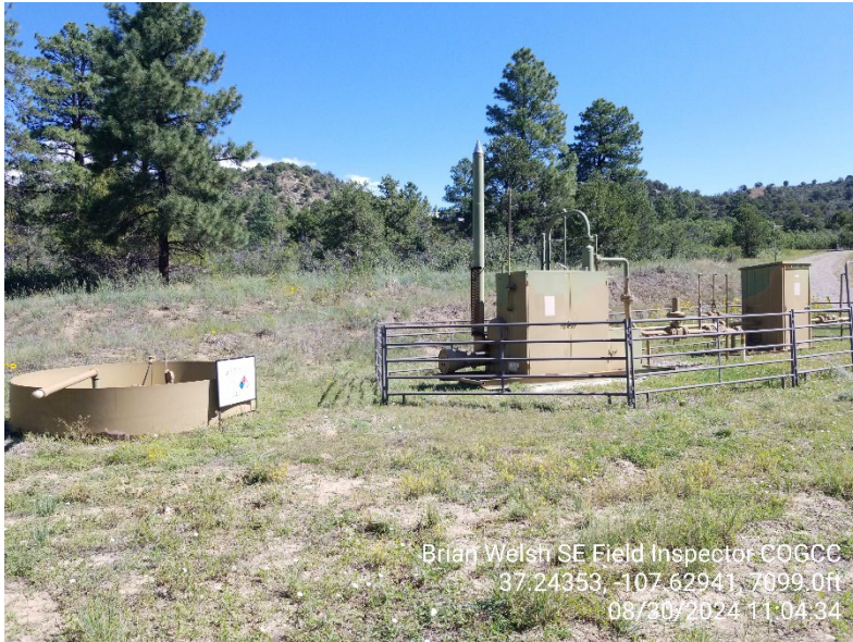
3. Production equipment and water tank
