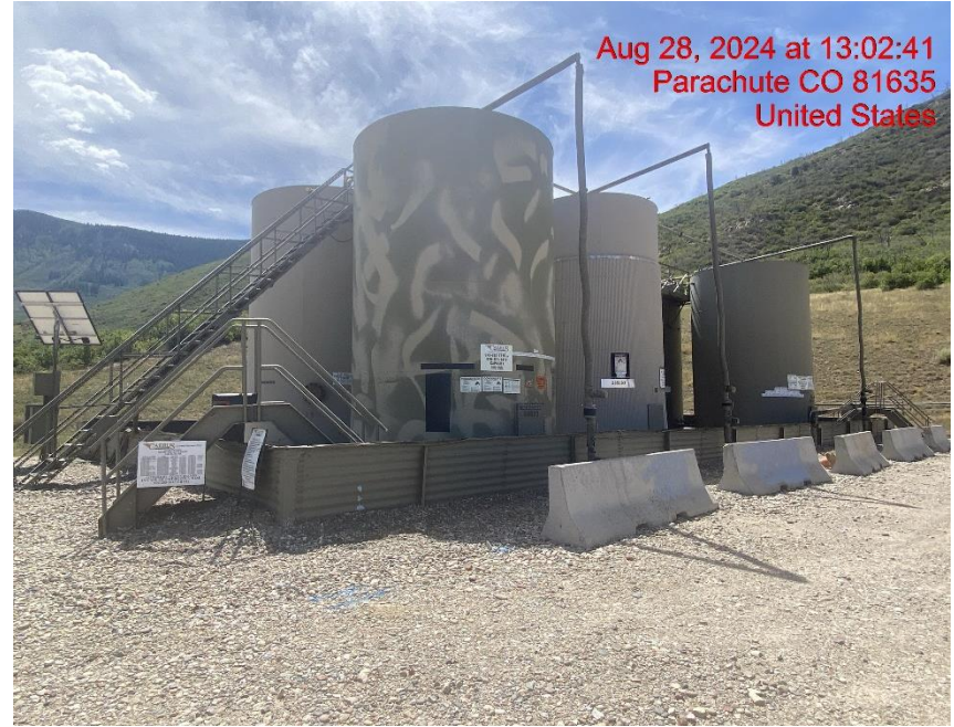
Tank Battery – Photo #03096
