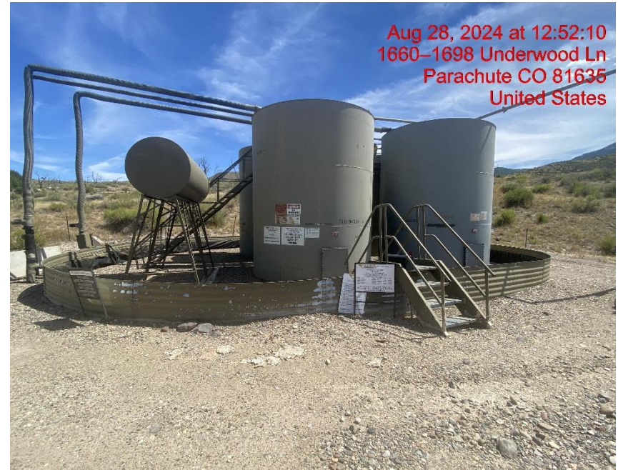
Tank Battery – Photo #03086
