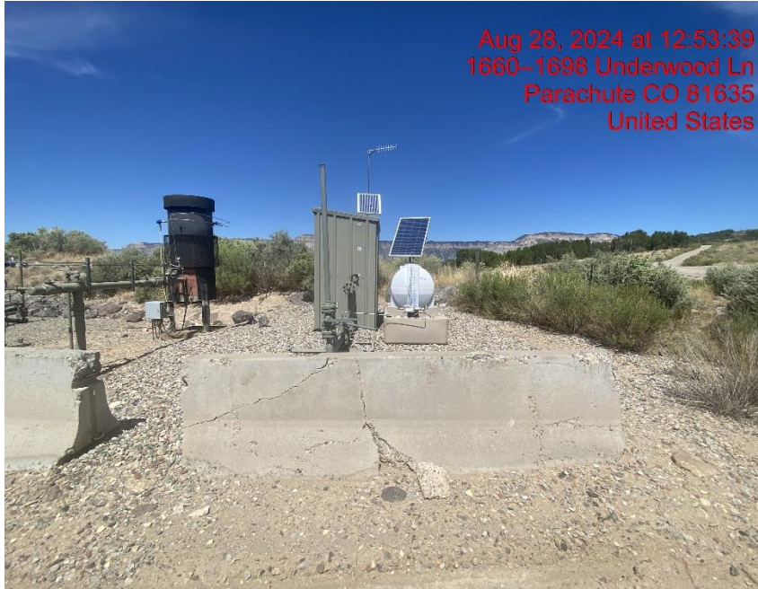
ECD/Gas Meter – Photo #03089
