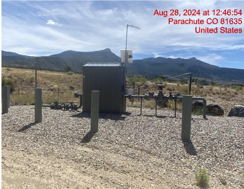
Gas Meter – Photo #03083
