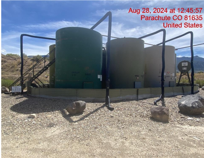
Tank Battery – Photo #03080
