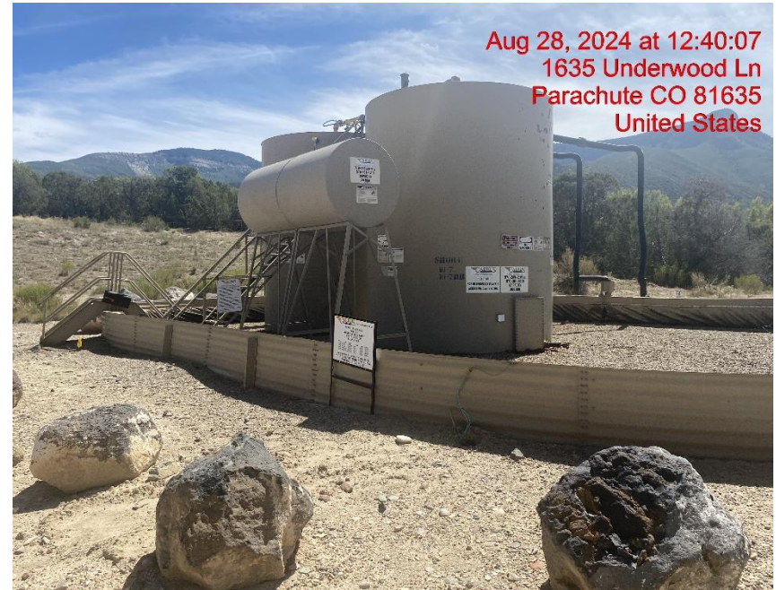
Tank Battery – Photo #03073
