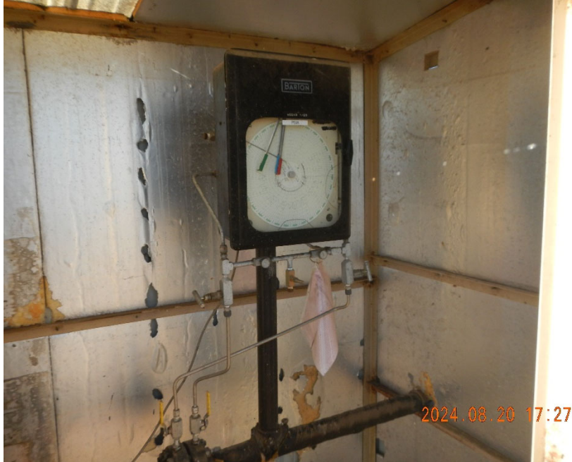
3. Gas meter inside meter shed.
