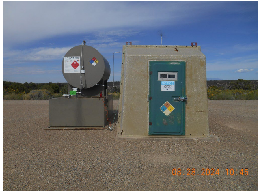
Injection wellhead housing Secondary containment of chemicals
