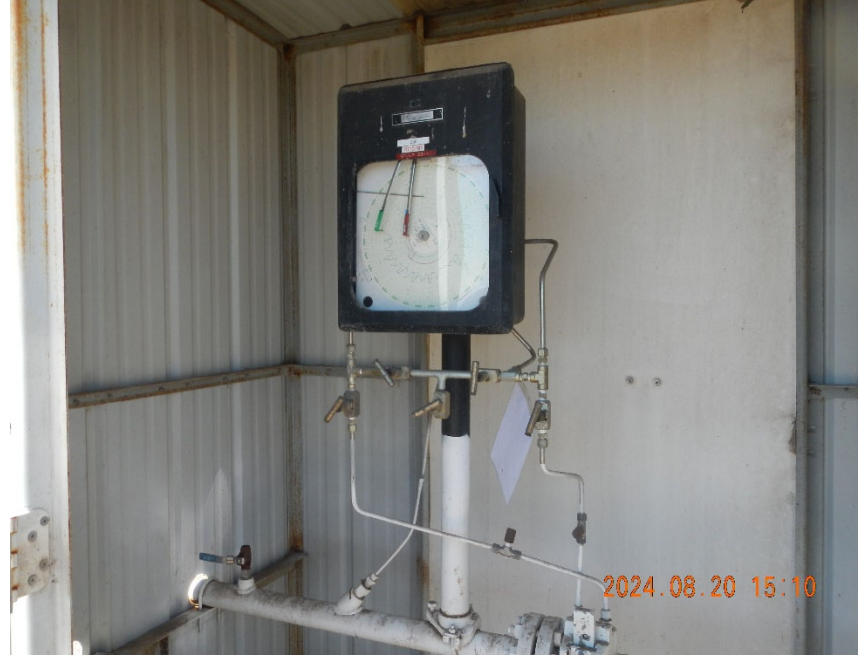
4. Gas meter inside remote meter shed.
