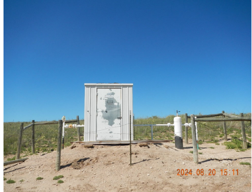
6. Remote battery overview.
