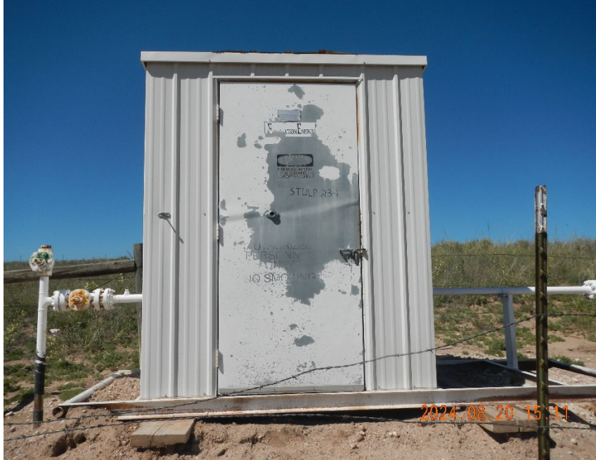
5. Remote meter shed.
