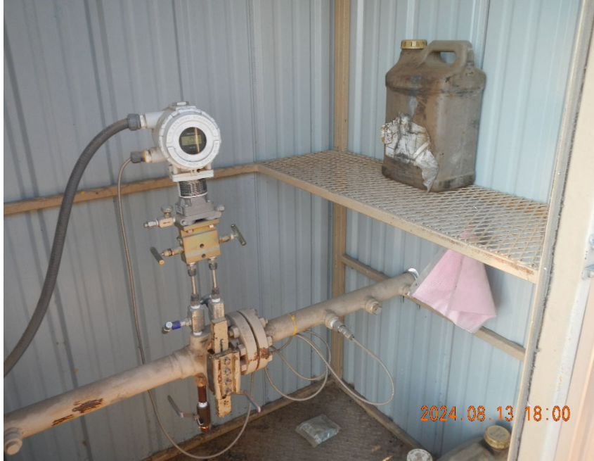
5. Gas meter inside remote meter shed.
