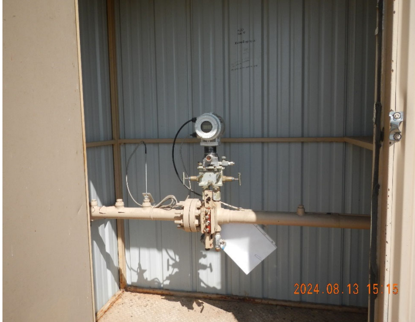
3. Digital gas meter inside meter shed.
