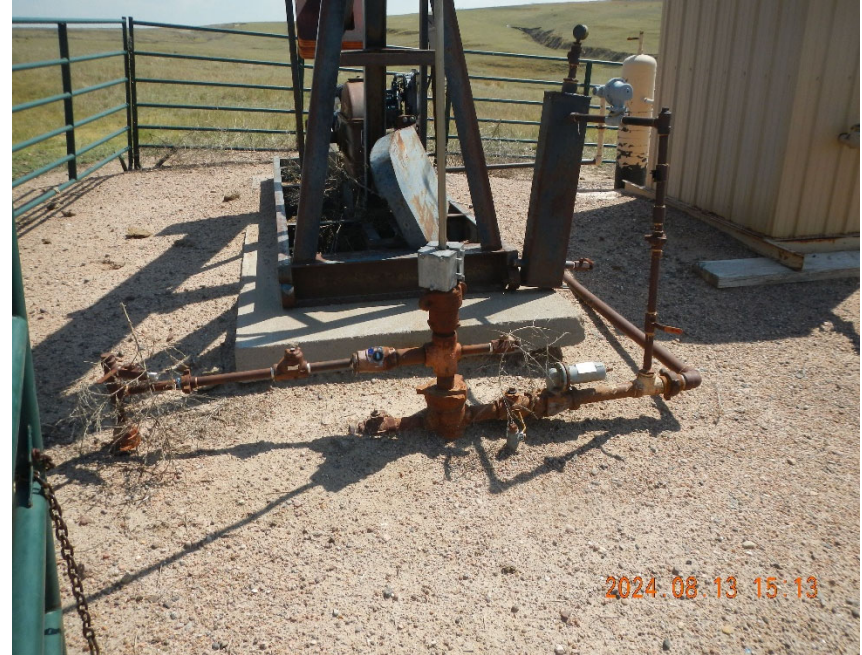
2. View of wellhead.
