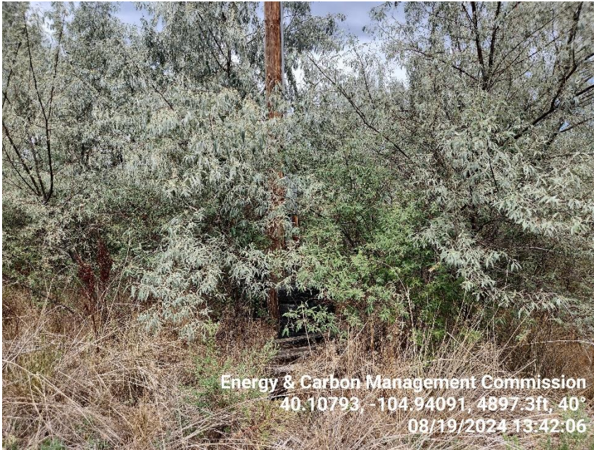
Photo 5 Ancillary equip. overrun with vegetation
