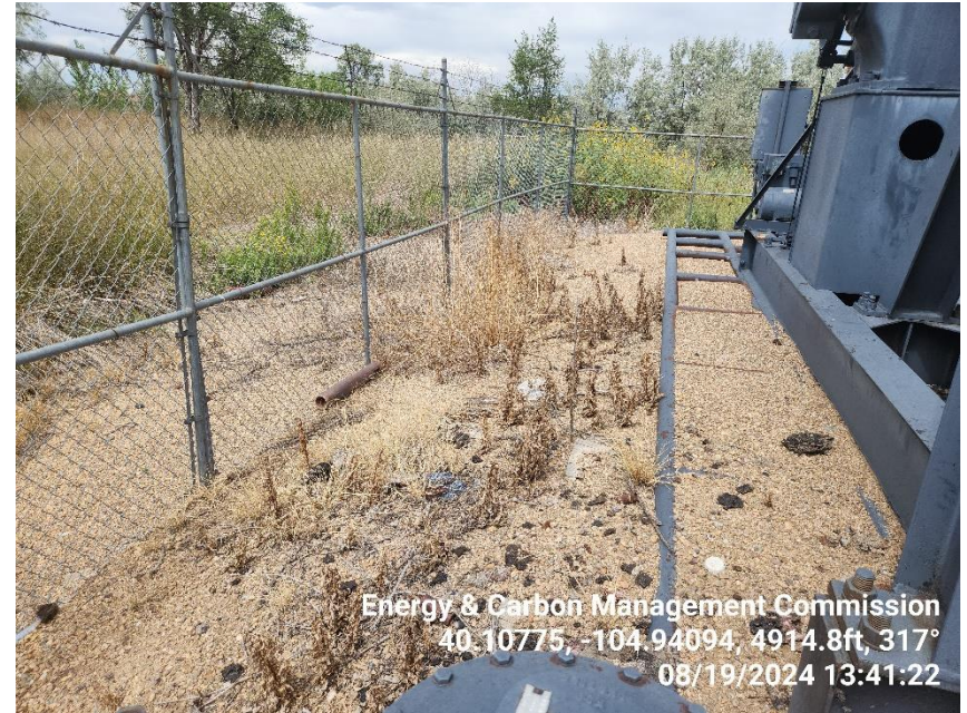
Photo 6 Dead vegetation & trash inside the wellsite fencing.
