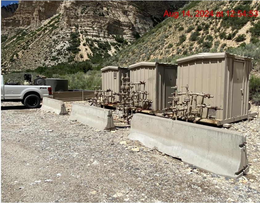
Gas Meters/Tank Battery – Photo #02828
