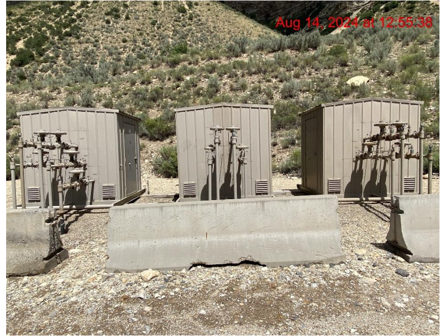
Gas Lift – Photo #02830
