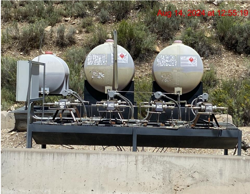
Chem Tanks – Photo #02829
