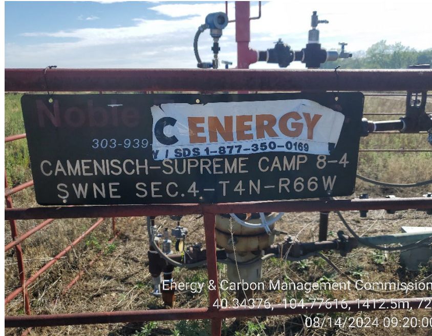
Wellhead and sign
