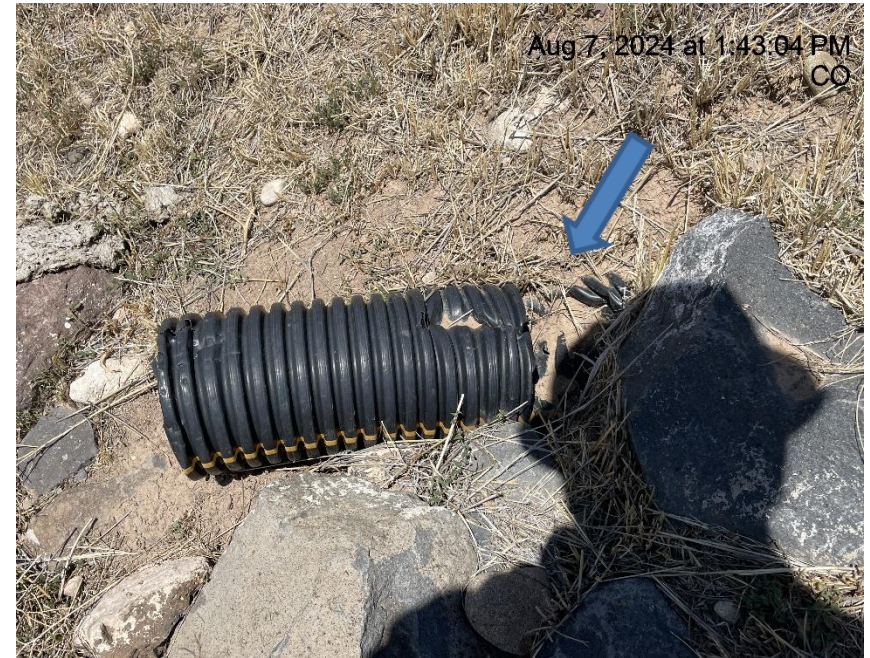
Photo # 5221 Drain line showing some signs of damage/needs maintenance
