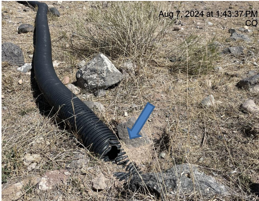
Photo # 5220 Drain line showing some signs of damage/needs maintenance
