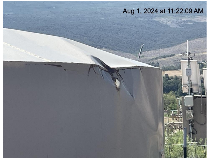
Photo # 4356 Production tank damaged
