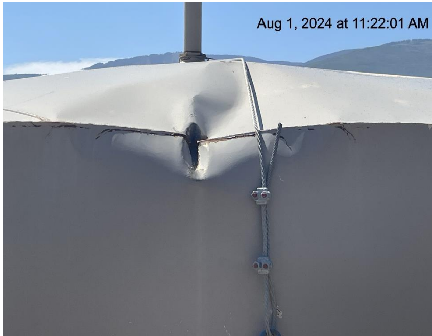
Photo # 4355 Production tank damaged
