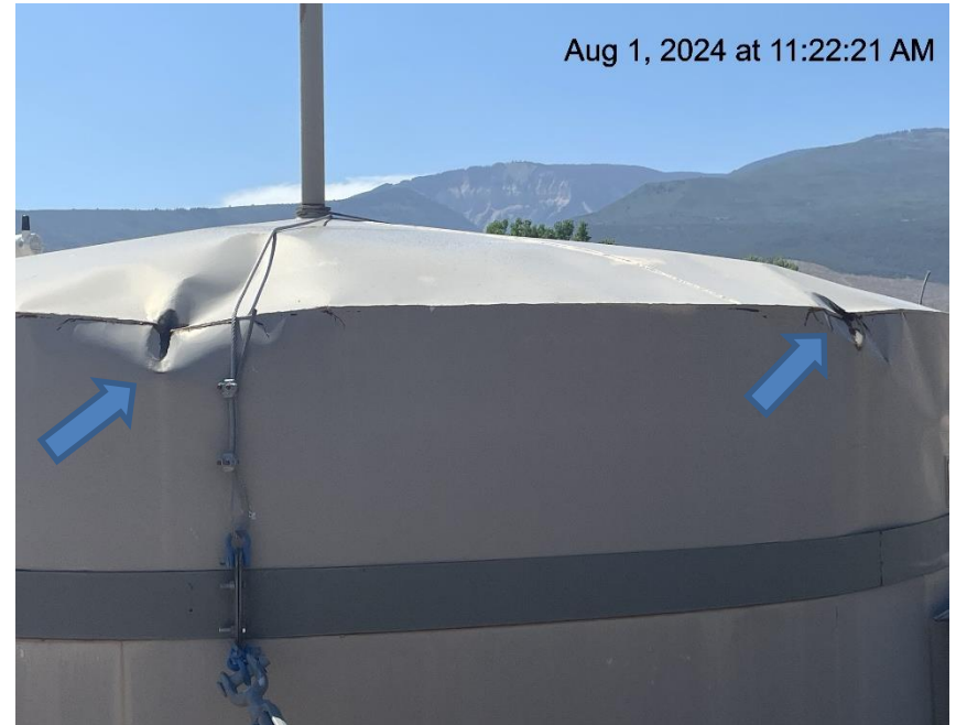
Photo # 4354 Production tank damaged
