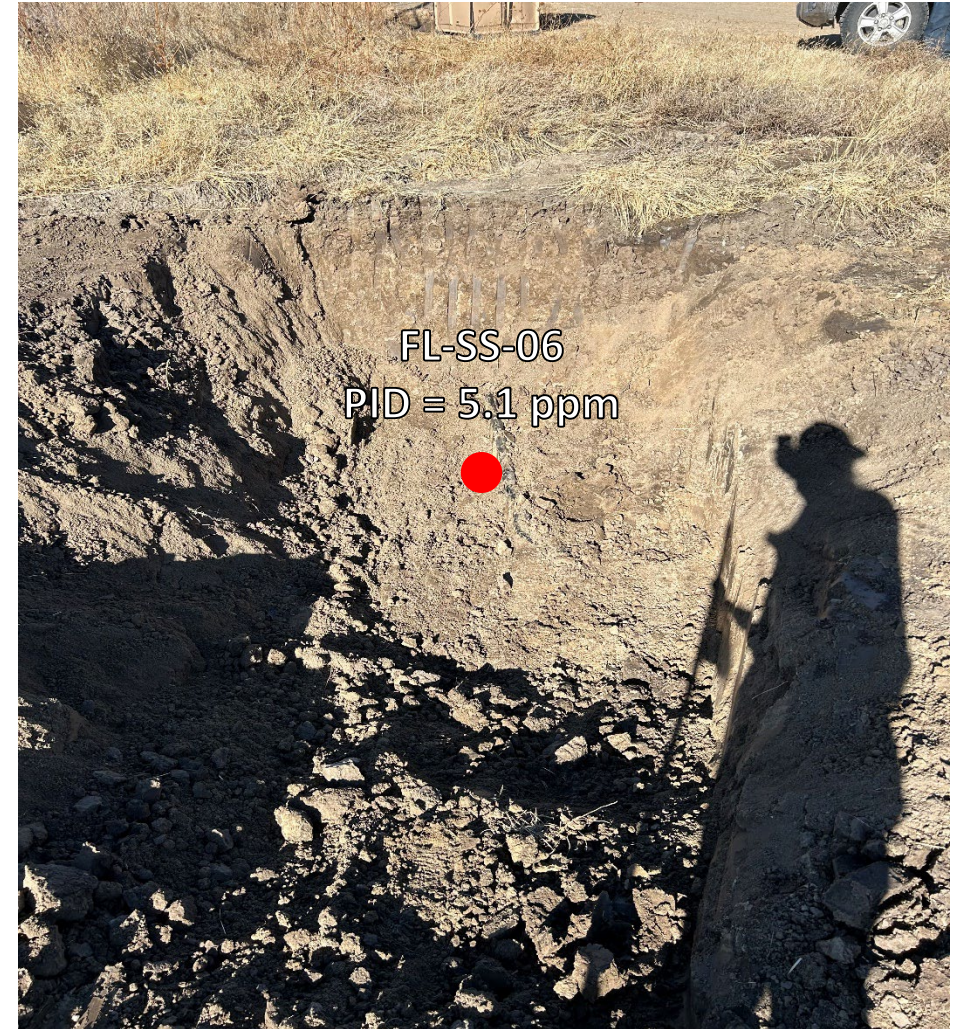
Looking north at flowline directional change
