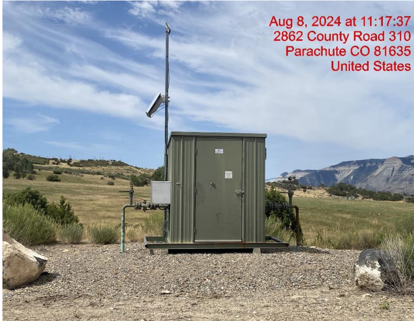
Gas Meter – Photo #02727
