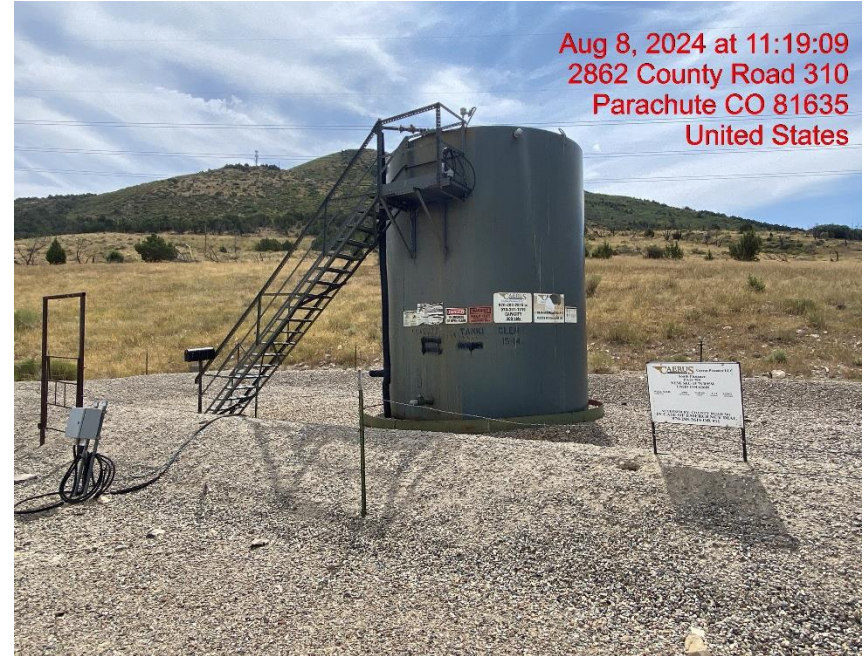
Tank Battery – Photo #02731
