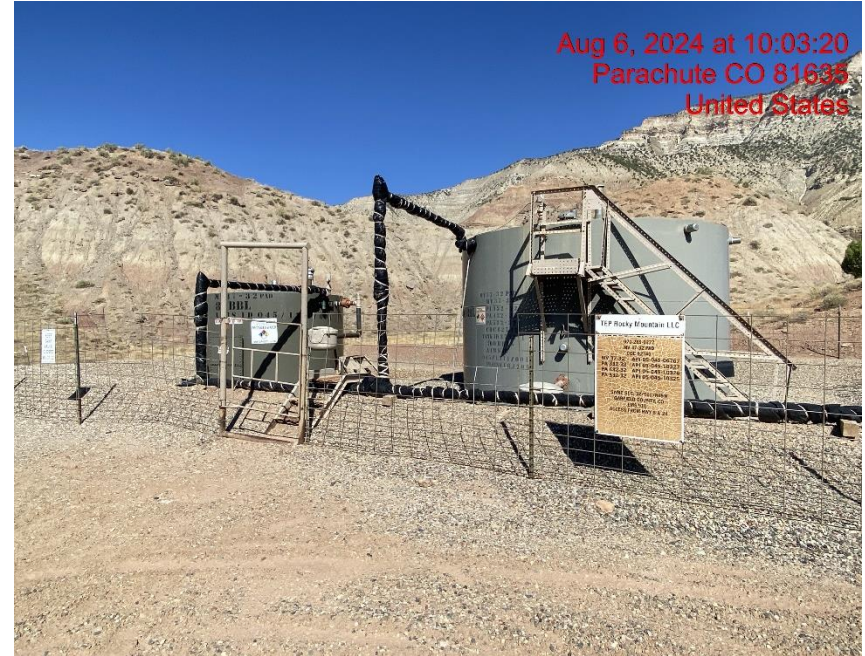
Tank Battery – Photo #02672
