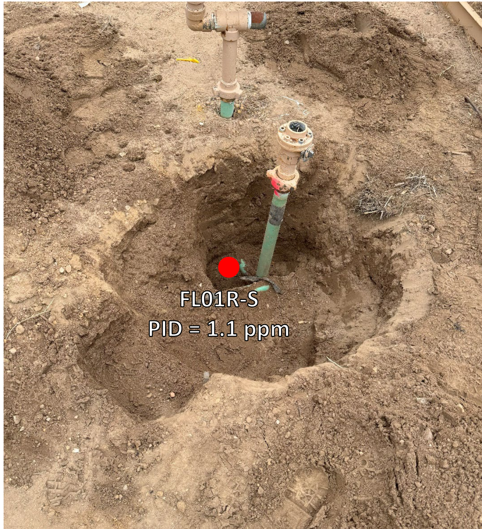
Looking west a flowline Pt B/terminus at separator No petroleum hydrocarbon staining or odor observed
