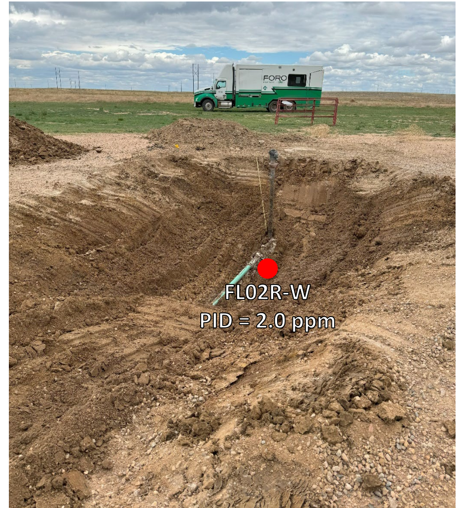
Looking west at Pt. A/terminus at wellhead No petroleum hydrocarbon staining or odor observed
