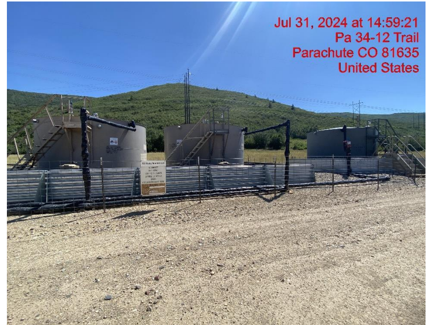
Tank Battery – Photo #02642
