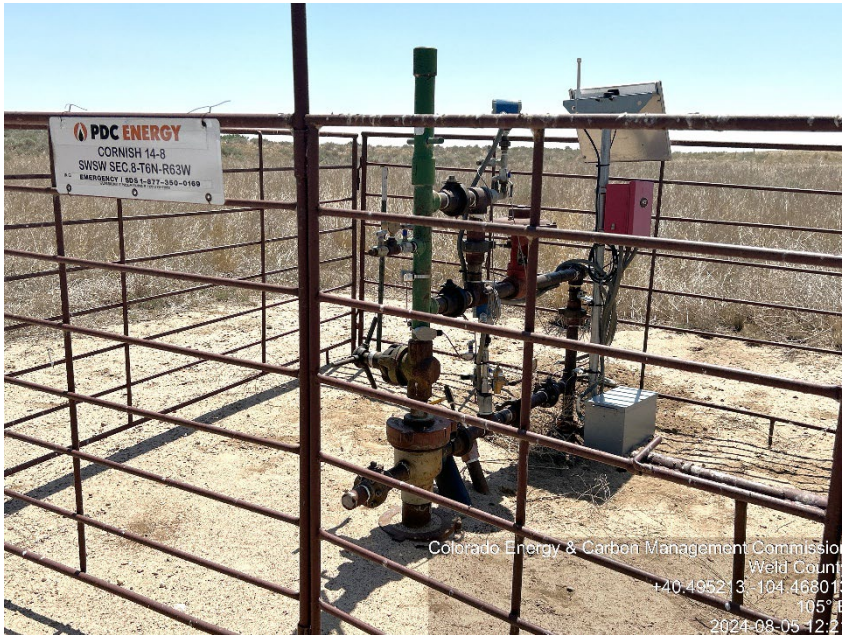
Photo #1 Cornish 14-8 (123-24168) Wellsite Producing | PR
