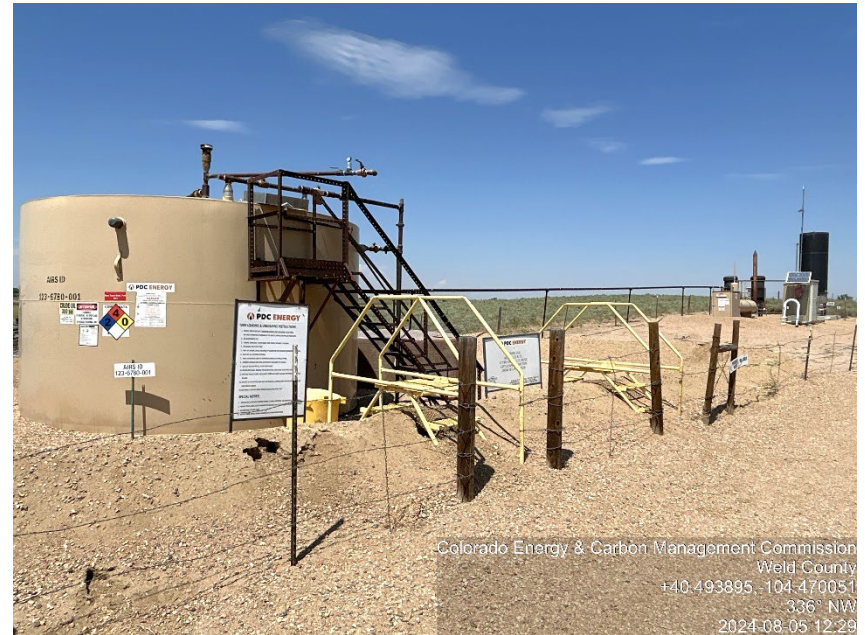
Photo #2 Cornish 14-8 Battery site Active Equipment Documented; Loc ID: 306191
