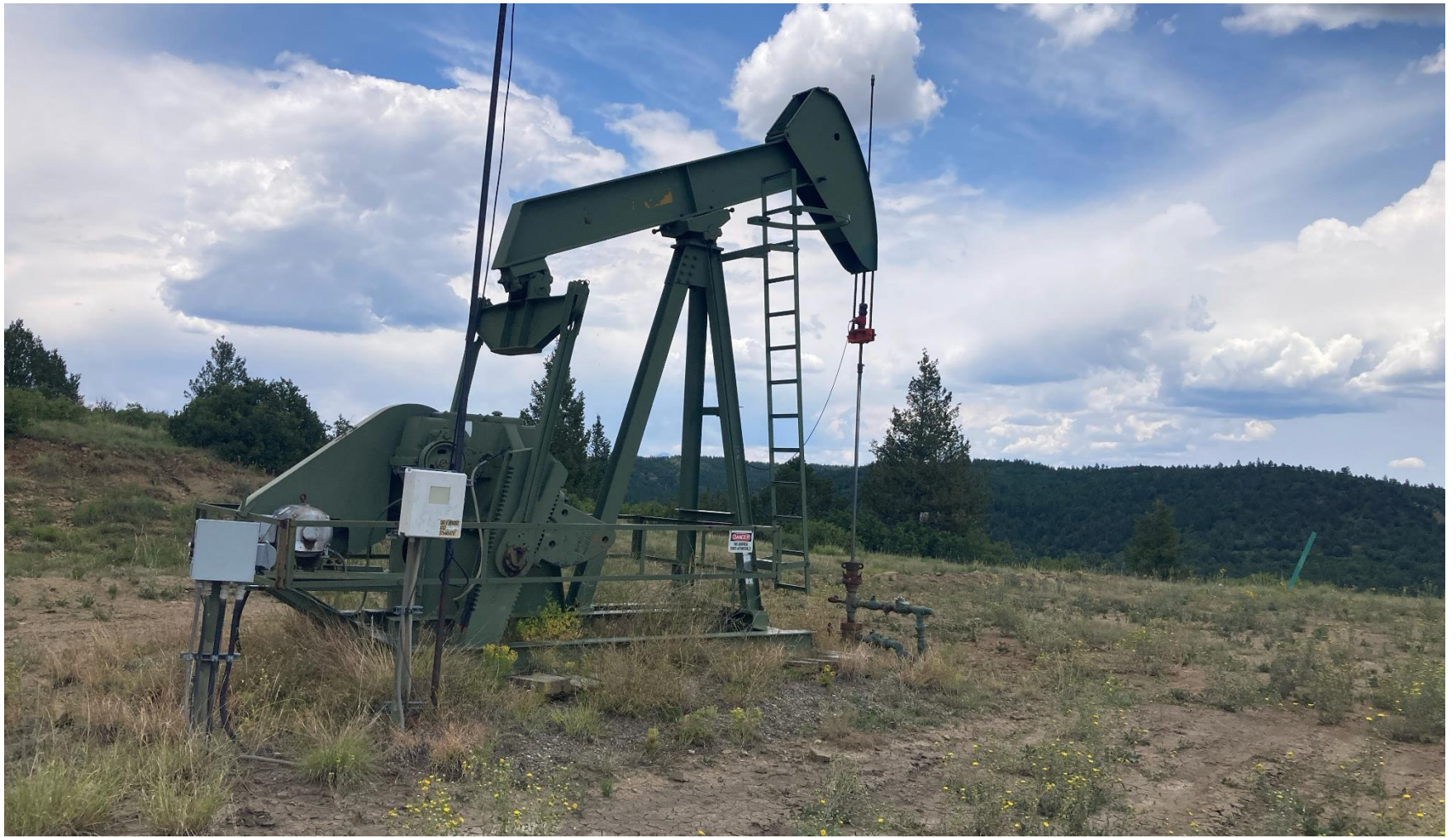
PHOTO 3: WELLHEAD AND EQUIPMENT
