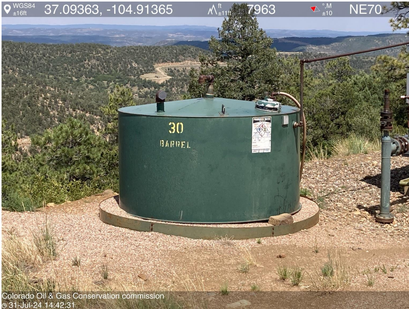
PHOTO 4: 30 bbl tank battery
