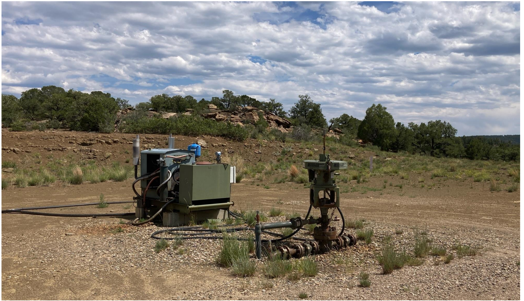
PHOTO 3: WELLHEAD AND EQUIPMENT
